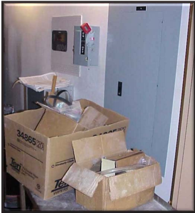
Improper Storage in front of Electrical Panel
