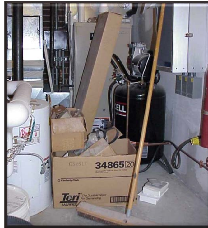
Improper Mechanical Room Storage
